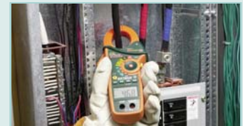
Collecting current measurements and associating them with the right component identified on an infrared image, can be a complicated and cumbersome process
